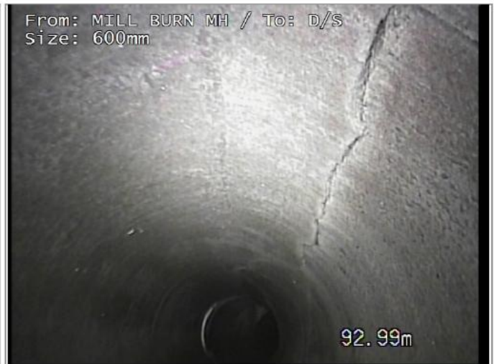
Crack longitudinal at 1 o'clock
