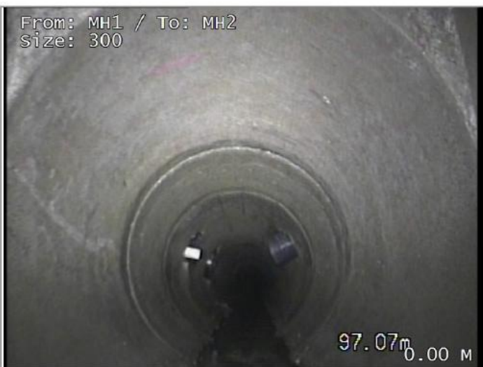
Finish node type, manhole, reference MH2 (Cover Buried)
