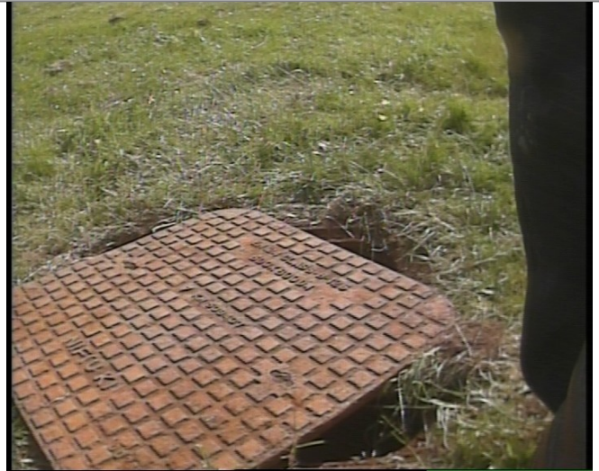
POINT B CP MH Location
