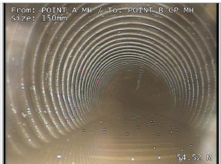
Survey abandoned - Remark: OUT OF CABLE, SURVEY WILL CONTINUE FROM POINT B CP BACK D/S.
