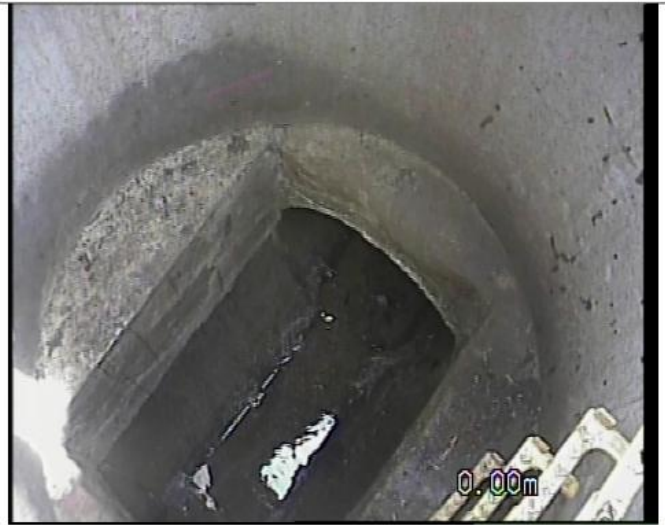
MILL BURN MH Internal
