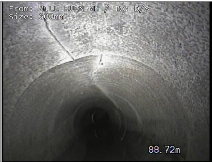
Crack longitudinal at 12 o'clock
