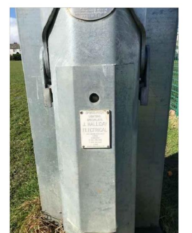
EXISTING ABACUS LIGHTING COLUMNS N.B. EXISTING LIGHTING COLUMNS ORIGINALLY INSTALLED BY HALLIDAY LIGHTING
