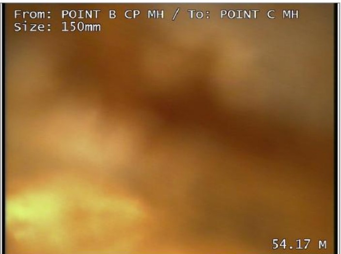
Survey abandoned - Remark: OUT OF CABLE, SURVEY WILL CONTINUE FROM POINT C MH TO POINT B MH
