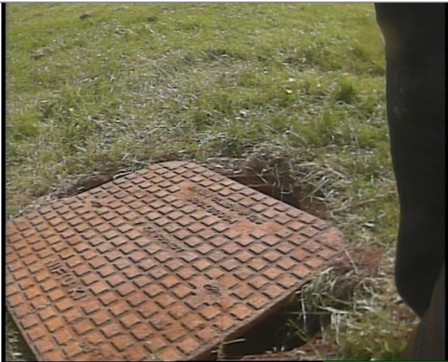
POINT B CP MH Location
