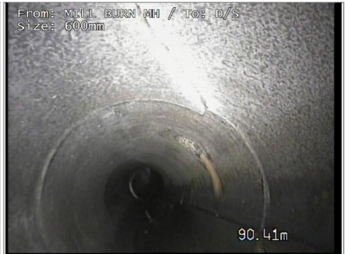
Crack longitudinal at 1 o'clock
