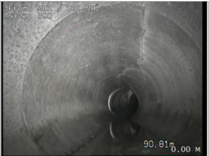
Crack longitudinal at 1 o'clock, Start
