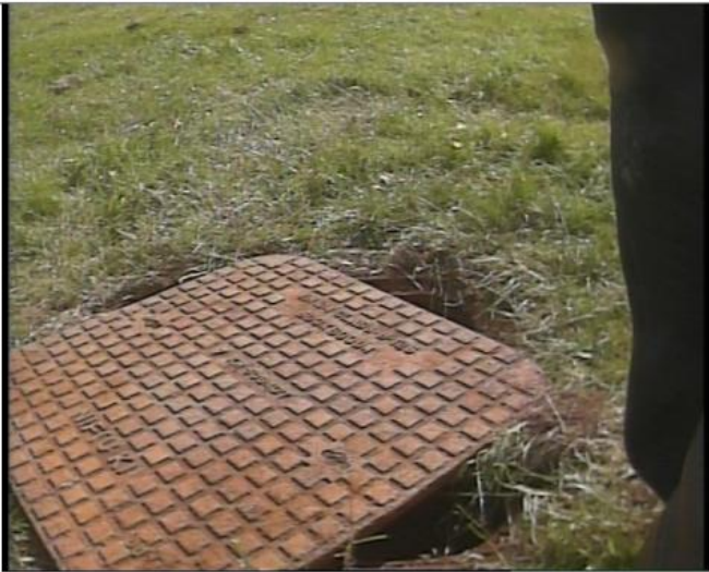
POINT B CP MH Location
