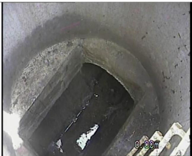
MILL BURN MH Internal
