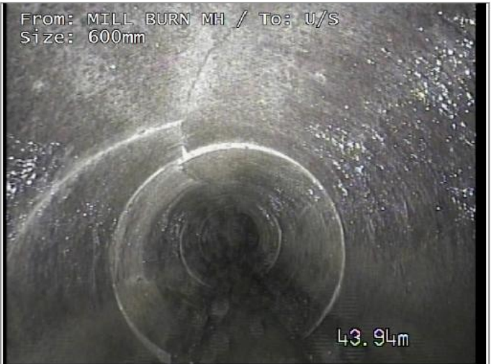
Cracks multiple from 12 to 9 o'clock
