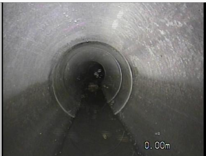
Start node type, manhole, reference MILL BURN MH
