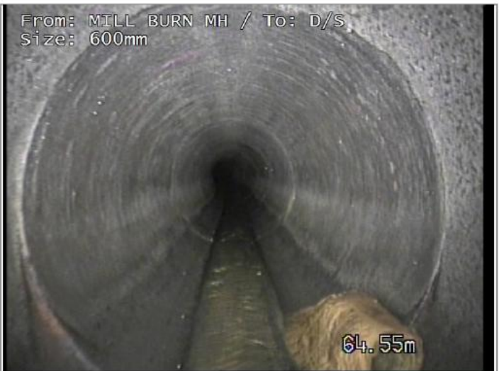
Attached deposits, encrustation at 5 o'clock 25% cross-sectional area loss
