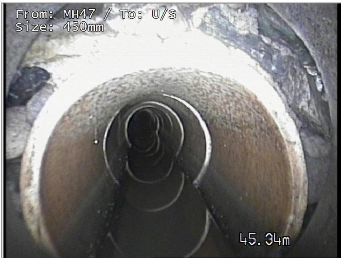
Survey abandoned - Remark: PIPE REDUCES, UNABLE TO PASS
