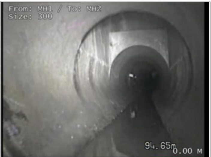
Crack longitudinal at 1 o'clock, Finished
