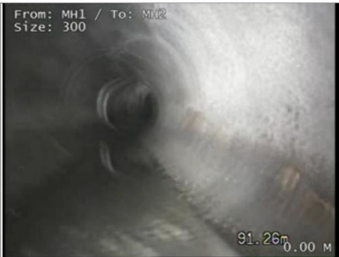
Settled deposits fine 5% cross-sectional area loss
