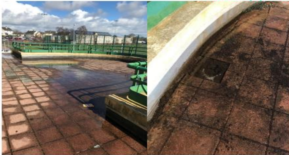
Standing water on terrace and blocked drainage outlet.
